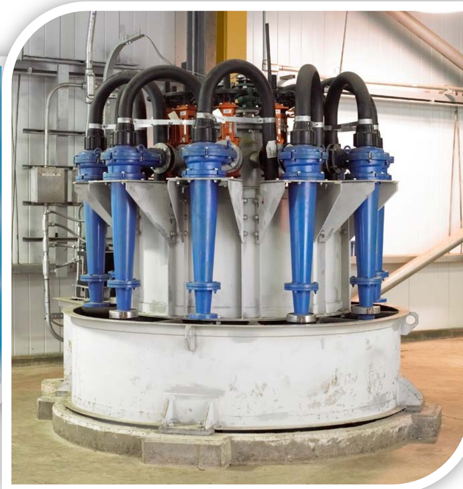
Primary Hydroclone Bank
