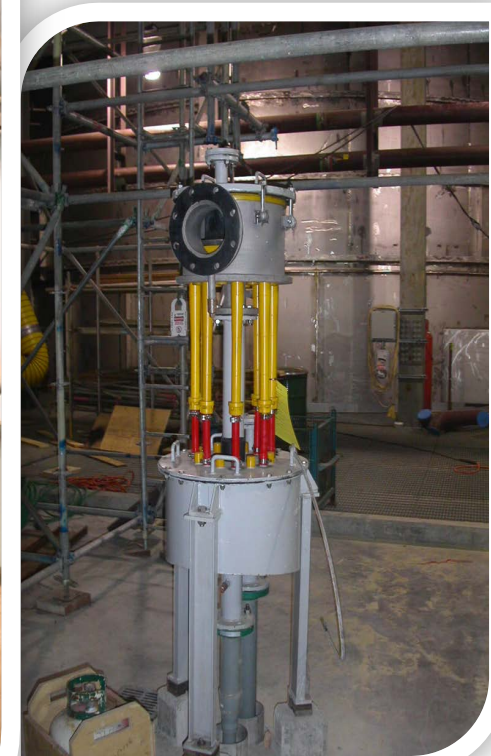
Secondary (Purge) Hydroclone Bank
